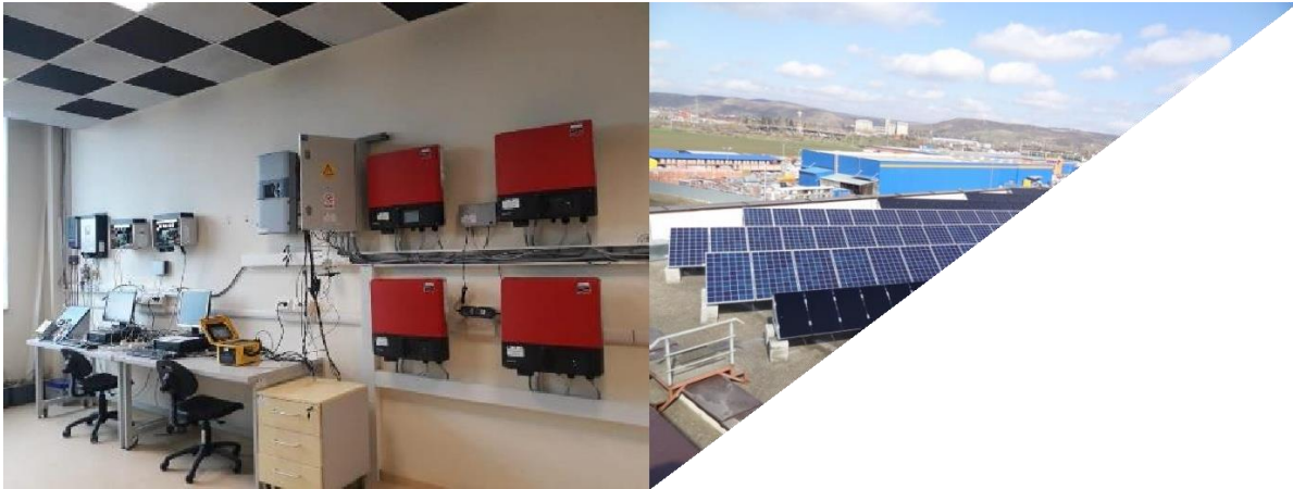
Photovoltaic experimental platform
